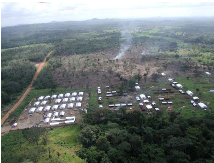
Largo camp under construction in 2002. Note the larger groups of reception area transit booths to the left of the picture, and then the smaller groups of transit booths between the communities in progress to the right of the picture. Note also, the smoke from the slash and burn clearance of ground in preparation of Phase 2. Image: Nicole
